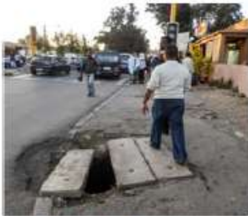
A) Poor Sidewalk
